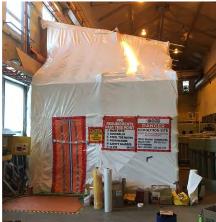
Figure D-1: Asbestos Containment Area
