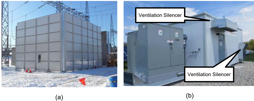
Figure 7-1 (a) Transformer Acoustic Enclosure (b) Inverter Enclosure with Silencers
