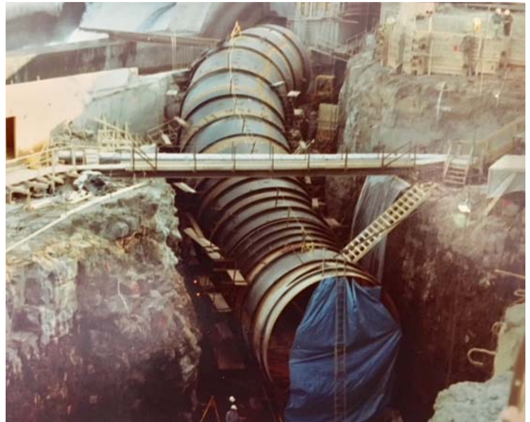
One of four penstocks at the Whitehorse Rapids Generating Station.
