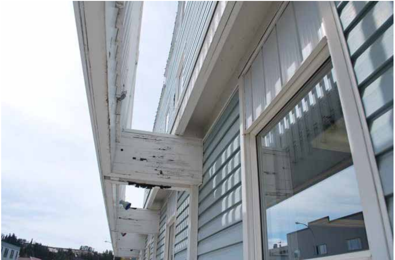
Photo 5 – Moisture damage on Glulam beams.
