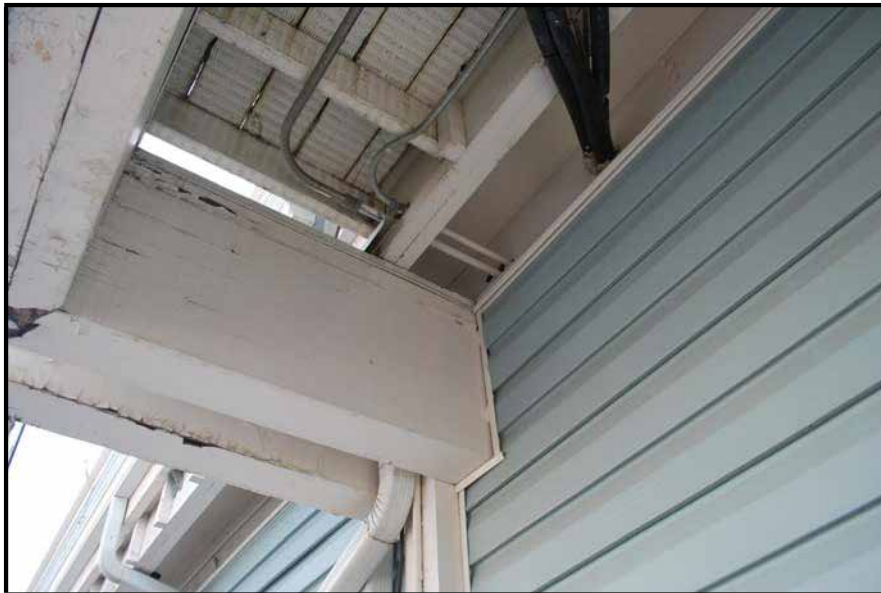
Photo 3 – Exterior Glulam beams at area of moisture leakage.
