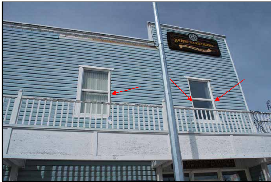
Photo 6 – Missing battens around windows.
