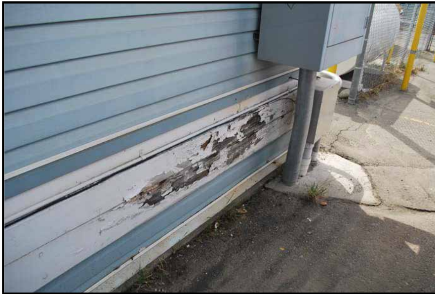
Photo 8 – Wood trim in poor condition.
