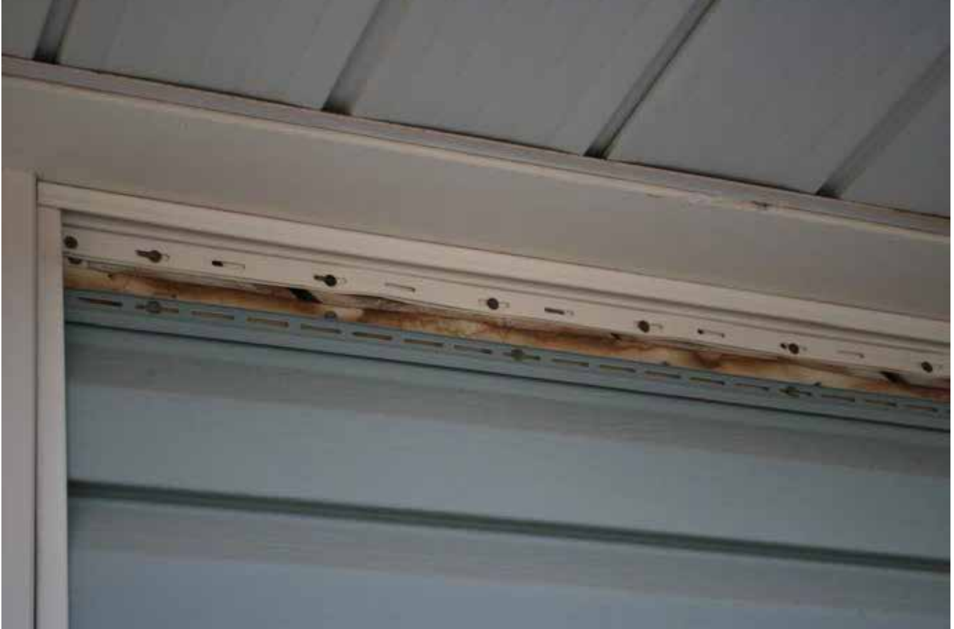
Photo 1 – Missing section of vinyl siding (moisture staining on wood sheathing).
