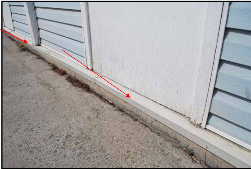
Photo 10 – Metal flashing sloping toward building allowing water to rest against wood trim.
