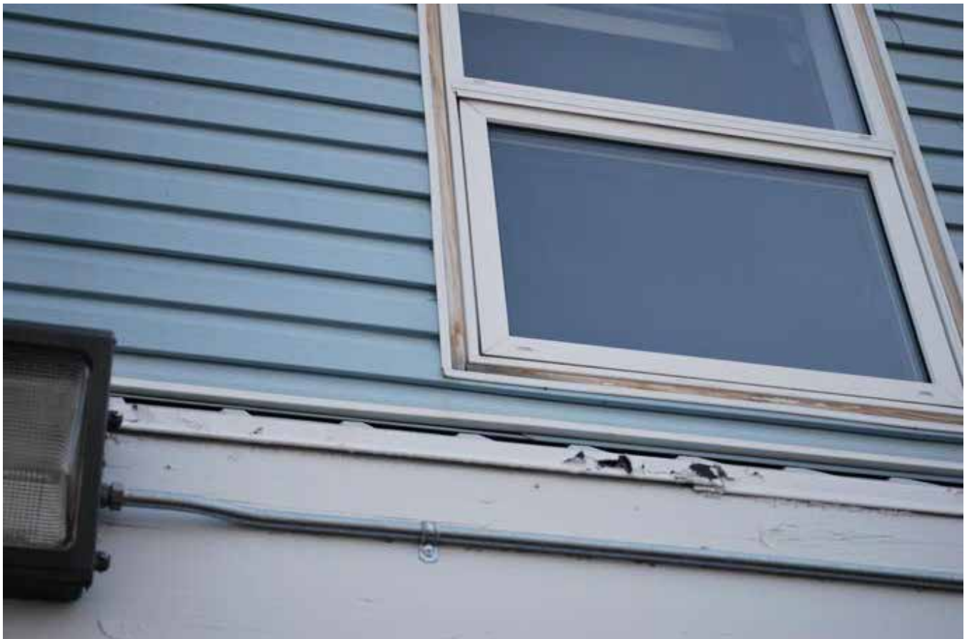
Photo 7 – Moisture staining on wood framing around window.
