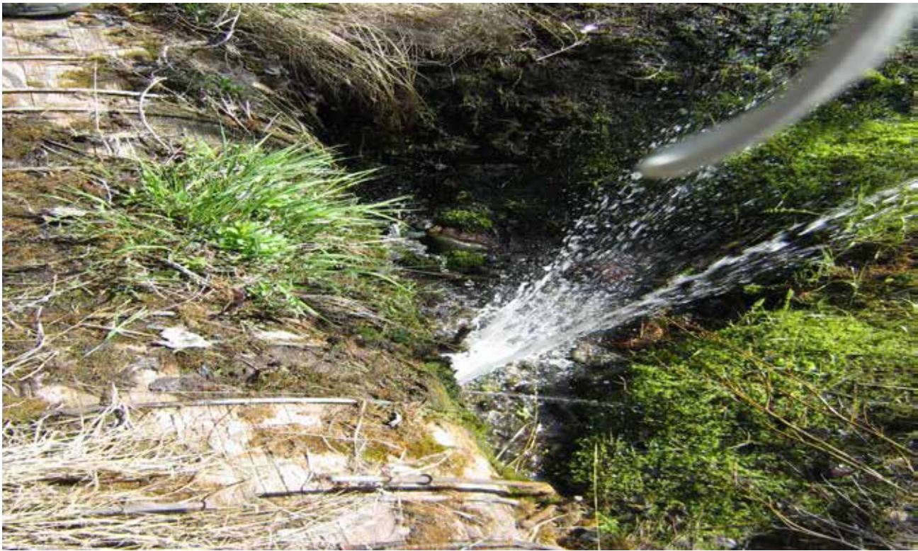
Figure 3 - Photo of Leak in Fish Lake Penstock #2
