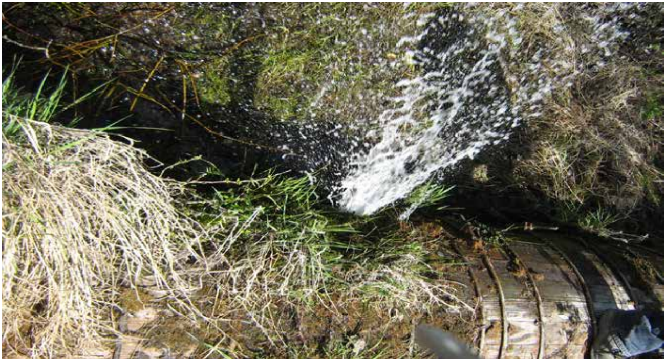
Figure 2 - Photo of Leak in Fish Lake Penstock #2
