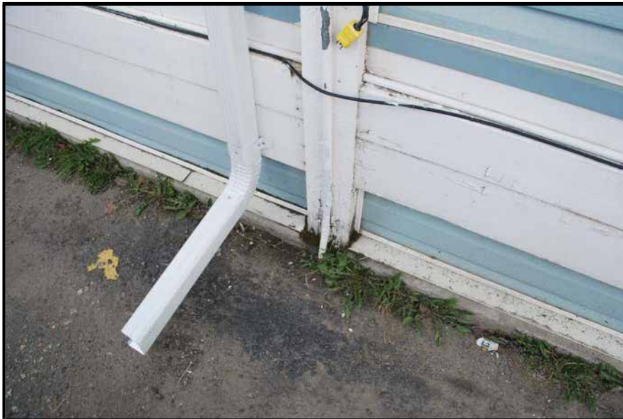
Photo 9 – Moss growth/moisture damage to wood trim/post.
