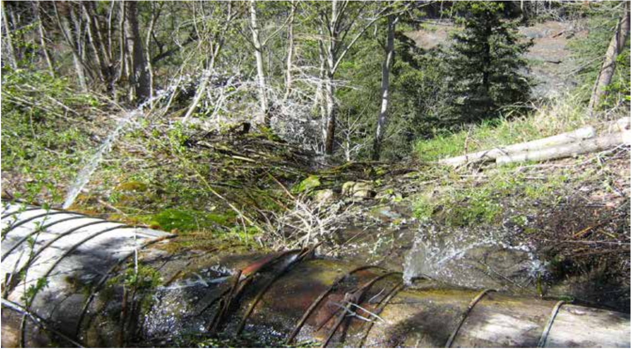
Figure 5 - Photo of Leak in Fish Lake Penstock #2
