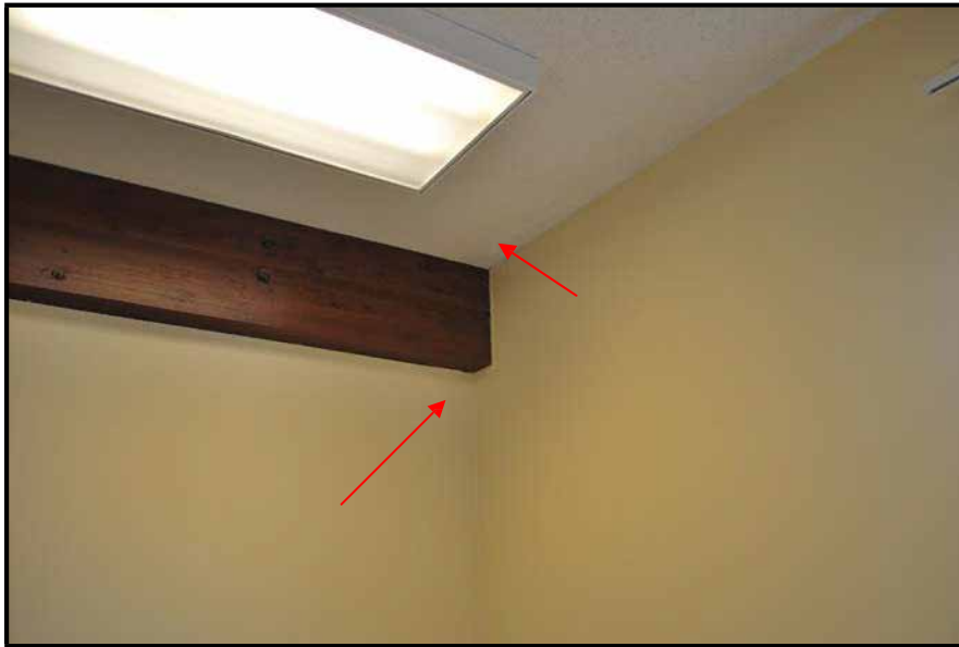
Photo 4 – Interior of Glulam beam at area of moisture leakage (water staining on ceiling, wall and in light fixture).
