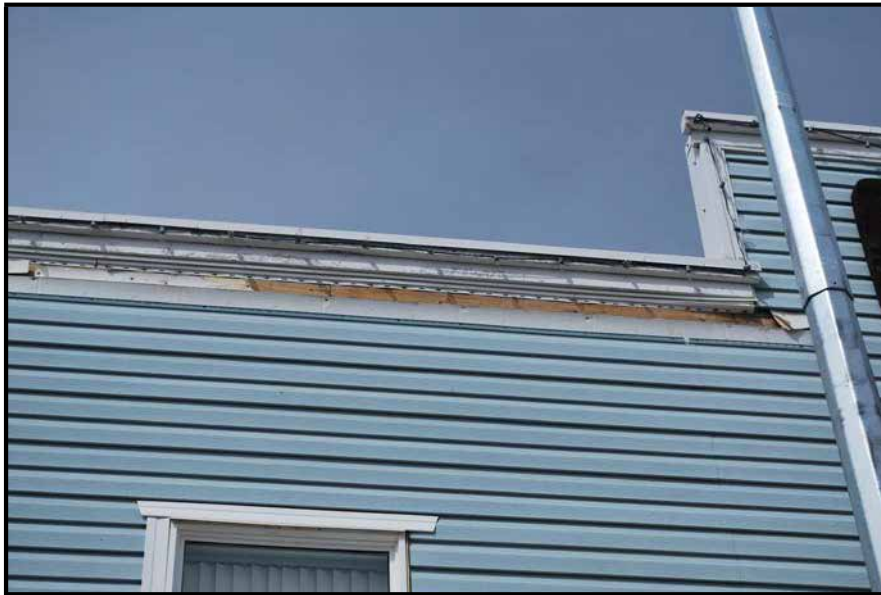
Photo 2 – Missing section of vinyl siding exposing wood sheathing.
