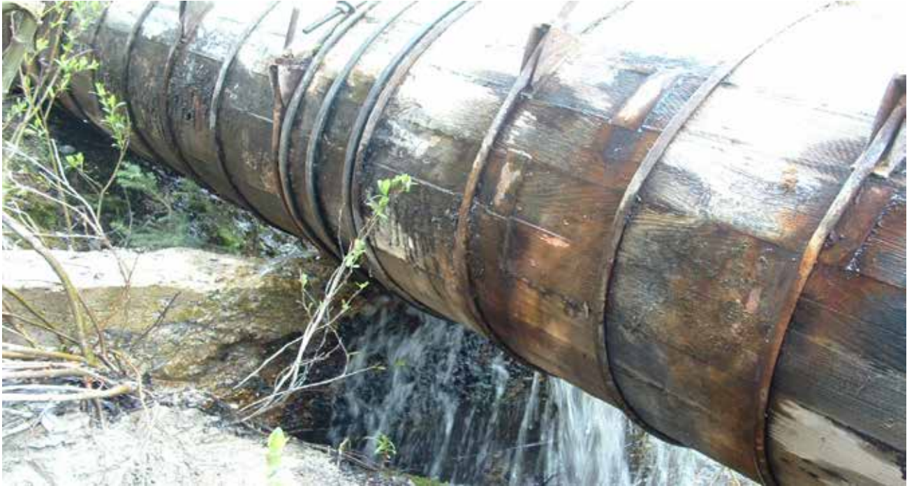
Figure 1 – Photo of Leak in Fish Lake Penstock #2
