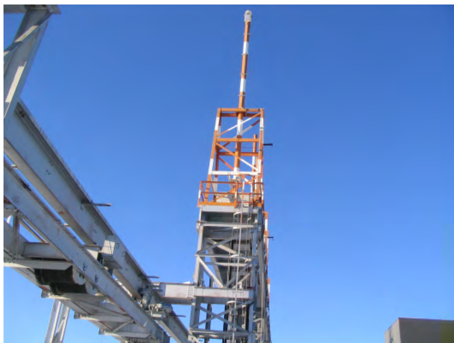
Pipe Sleeve / Drive Guarding and Support Structure
