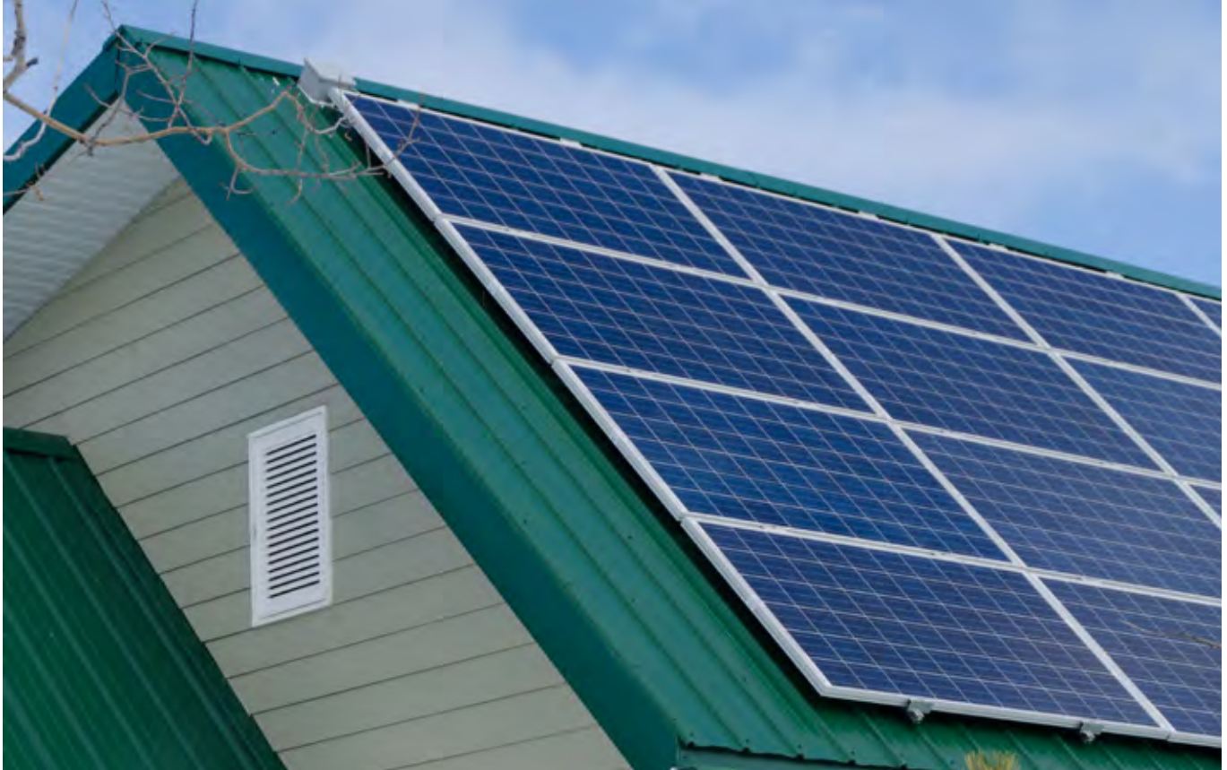
Home with solar panels.
