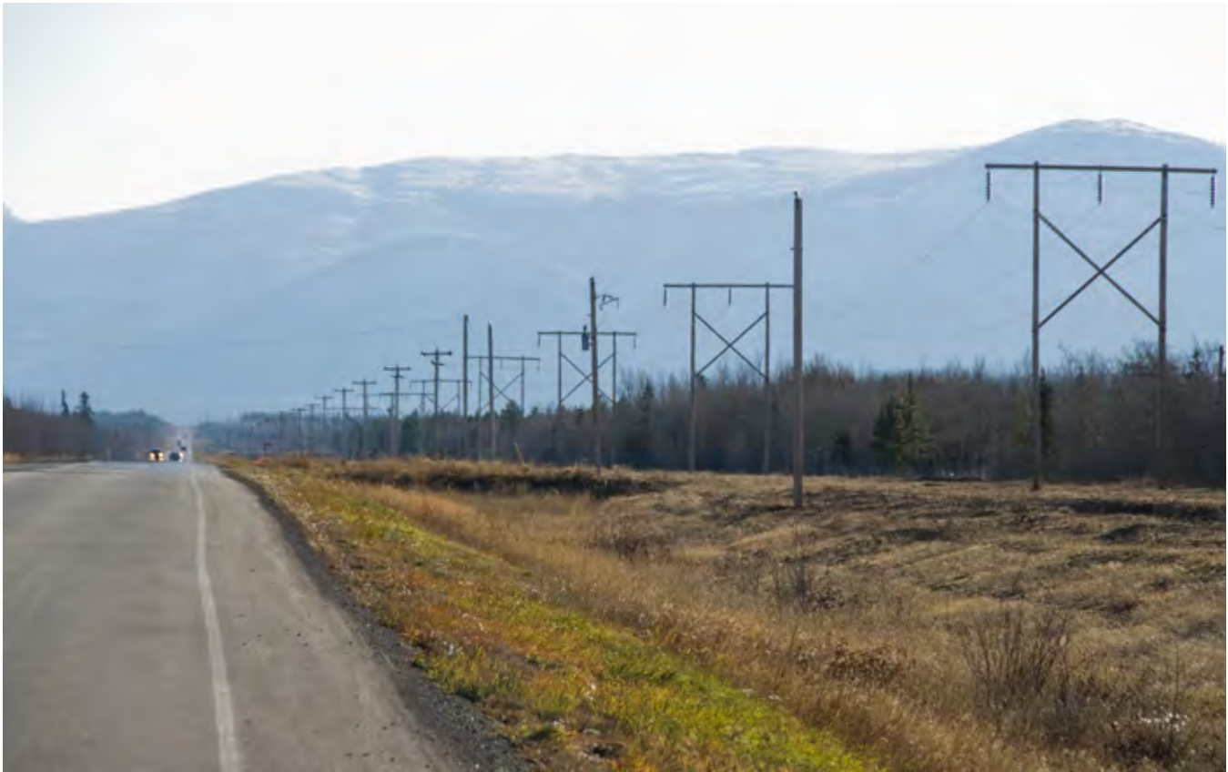
Power lines running along highway.
