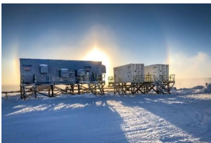
Battery Energy Storage System in the Arctic
