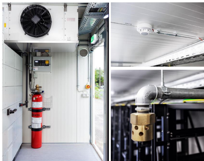
Figure 4-5: Sample of fire protection system, showing pressurized container of fire suppressant on left side, the fire/smoke detector in the container on the upper right, and the nozzle for dispensing the fire suppressant if required, on the bottom right.
