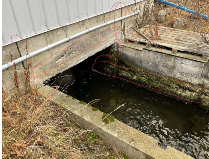
Figure 26: degraded concrete on tailrace walls
