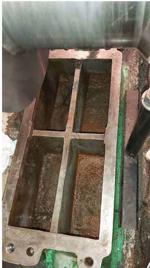
Figure 8: Turbine Bearing Pedestal Hole to Ground
