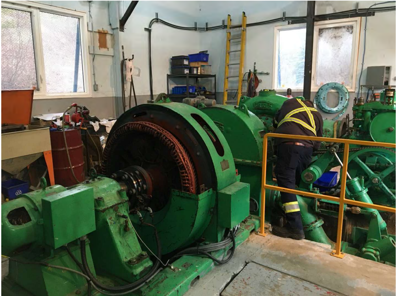
Figure 1: Turbine and Generator
