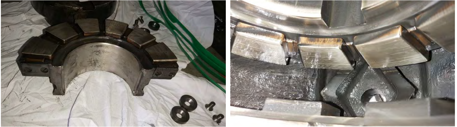
Figure 7: Thrust Pad Damage
