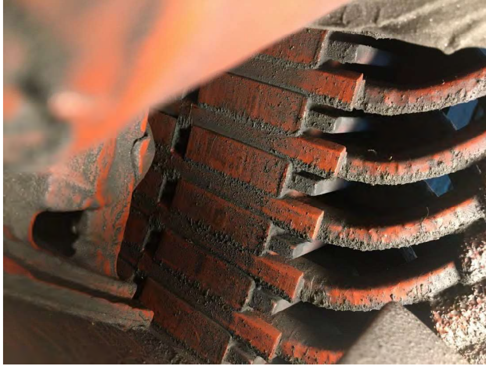
Figure 12: Stator and End Turns with Carbon Dust Buildup
