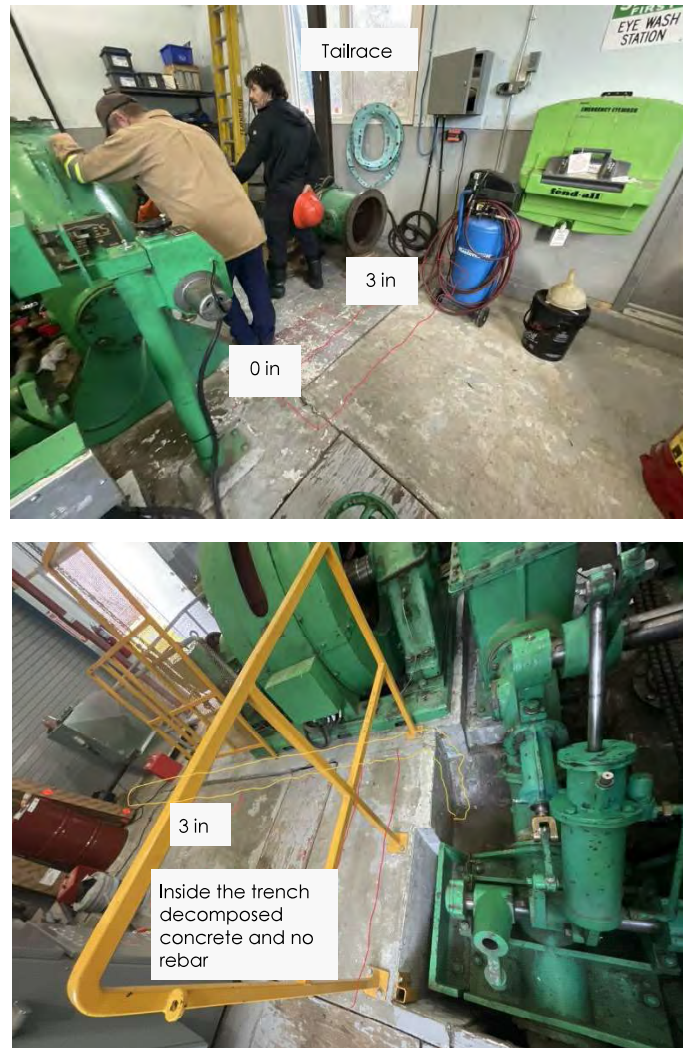
Figure 22: Differential settlement between the concrete block and slab on grade
