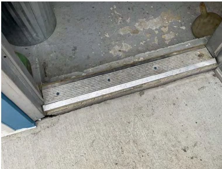
Figure 27: Differential settlement outside and inside the building
