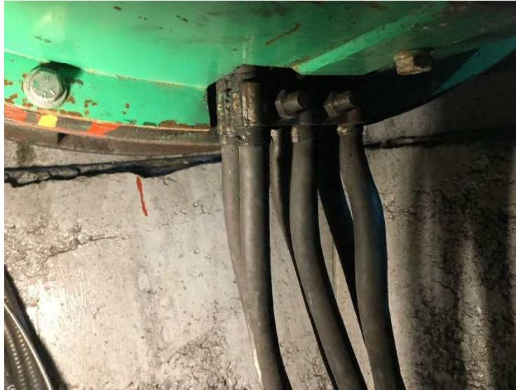
Figure 20: MV Cables Under Generator
