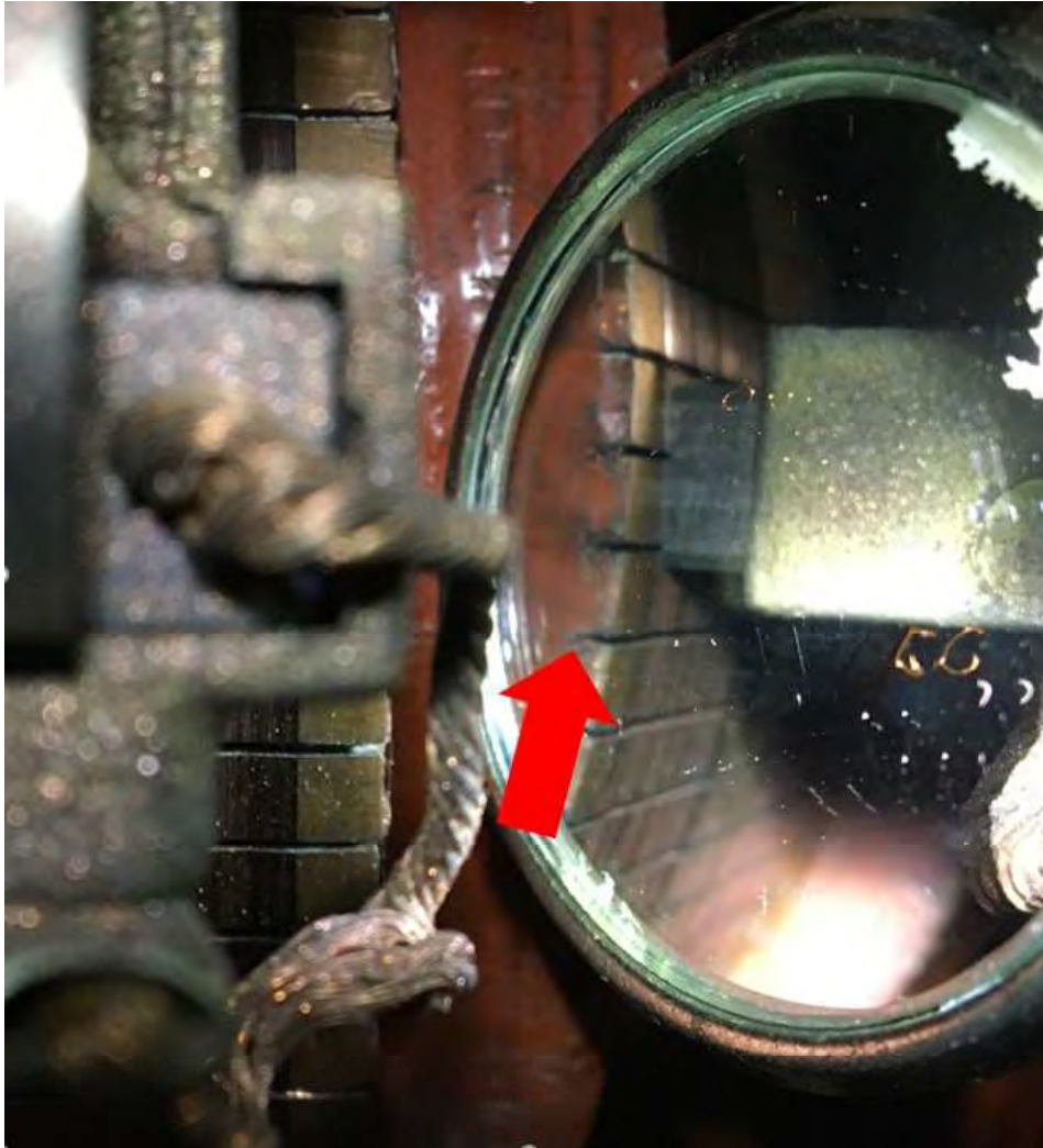
Figure 18: Commutator Remaining Surface (~3 to 4mm)
