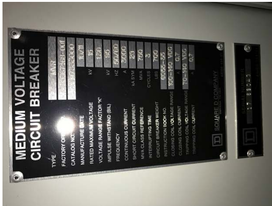
Generator Circuit Breaker Nameplate
