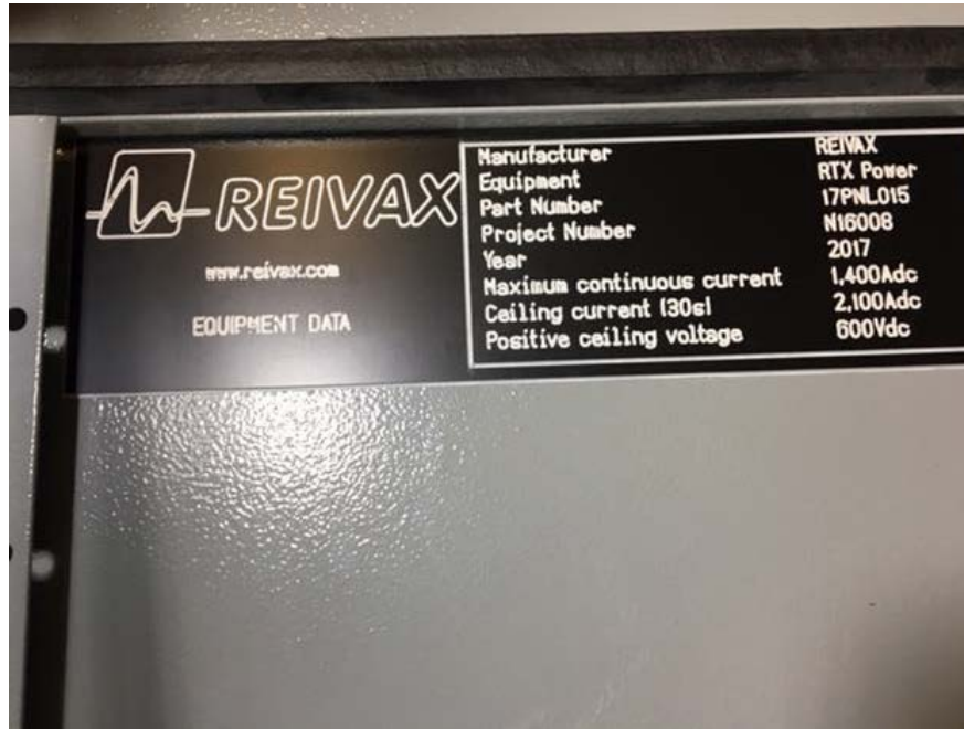
Excitation System Nameplate
