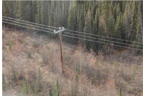
Figure 13. Less than 3 meters clearance, L 250 spans 105-106.
