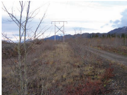
Figure 9. Typical ground view of ROW showing ground and edge conditions, no maintenance required at this time (Line L 170A).
