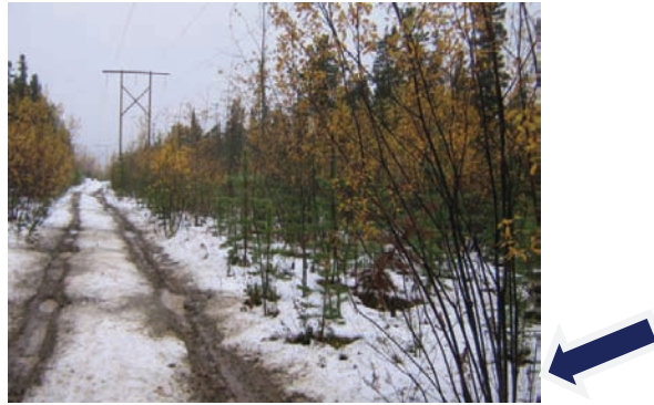
Figure 10. Typical ground view of ROW showing ground and edge conditions, maintenance required within 1 year (Line L 169). Note multiple stems re-sprouting from previously cut stump in lower right corner of photo.
